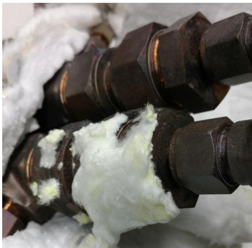
Figure 3-28 Pump outlet loop leg salt leak site
