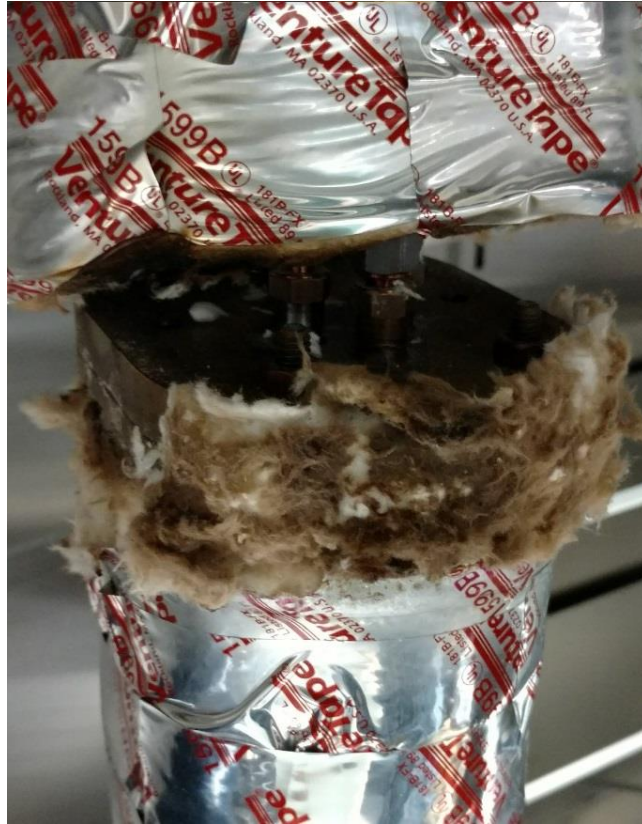
Figure 3-26 Salt leakage around expansion tank gasket
